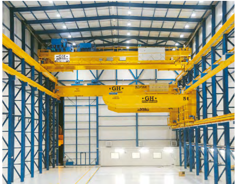
Double girder crane and cantilever crane
